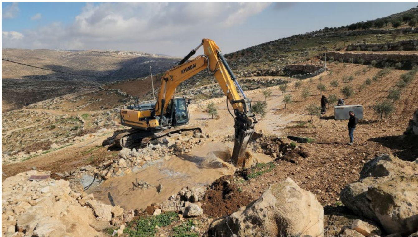
Demolition of a rainwater cistern in al-Buweib in the South Hebron Hills. Photo by Nasser Nawaj'ah, B'Tselem, 12 February 2023.
