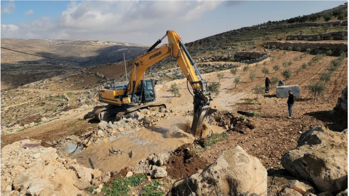
Demolition of a rainwater cistern in al-Buweib in the South Hebron Hills. Photo by Nasser Nawaj'ah, B'Tselem, 12 February 2023.
