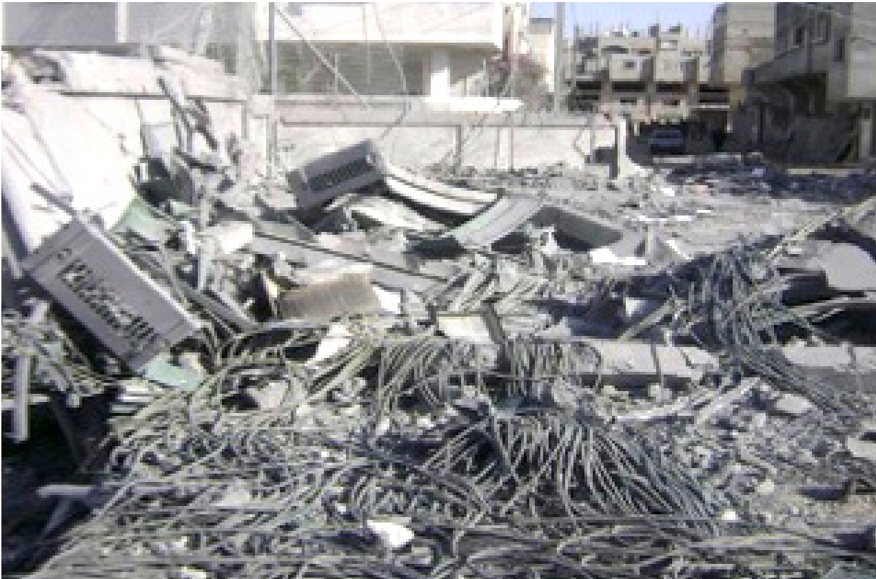
Paltel's main switch in North Gaza demolished on the first day of Israel's military assault | January 2009 | Photo: Paltel Group, Gaza Directorate
