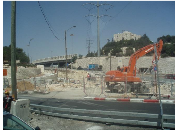
A DOOSAN TRACK EXCAVATOR DURING THE CONSTRUCTION OF THE JERUSALEM LIGHT RAIL, EAST JERUSALEM, AUGUST 2009. PHOTO BY WHO PROFITS.
