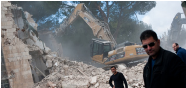
A Caterpillar excavator operated by Benny & Tzvika during the demolition of the Shepherd Hotel | Sheikh Jarrah, East Jerusalem | 9 January 2011 | Photo by Activestills
