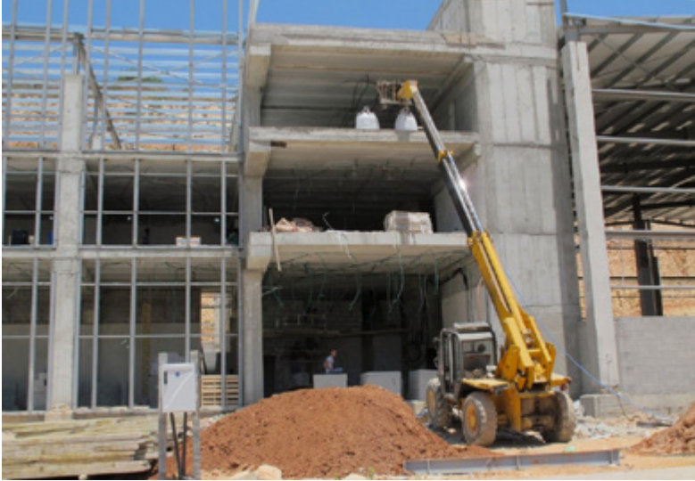
JCB machinery conducting construction work | Barkan Industrial Zone | 20 June 2013 | Photo by Esti Tsai
