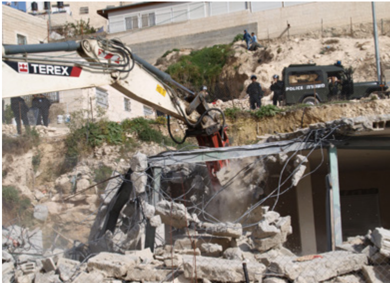
Terex machinery during a house demolition | At-Tur neighborhood, East Jerusalem | 8 February 2009 | Photo by L. Aarvik
