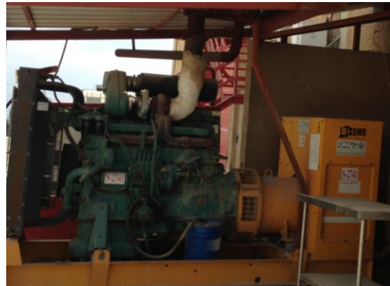
Photo no. 12: SDMO generator, provides by Shmerling-Synchro Energy Engineering in Ahava's production site | Mitzpe Shalem settlement | Who Profits | April 2013
